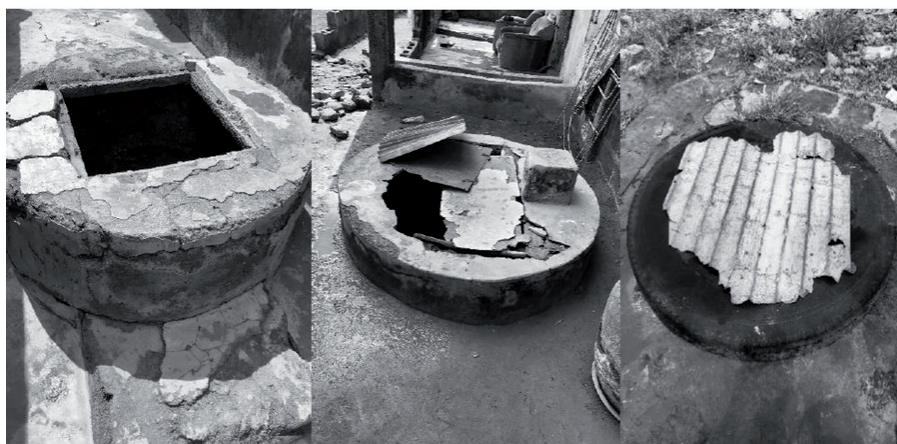
Fig. 2a). Poorly maintained hand-dug wells within the communities.
