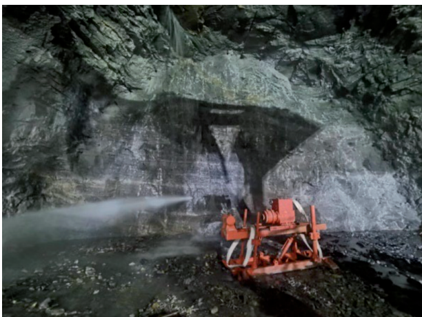
Fig. 2. Water inrush situation of the tunnel face.
